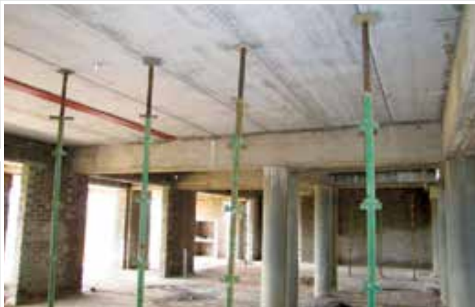
Centre line of props - One prop per panel. (Only for spans longer than 5m)
