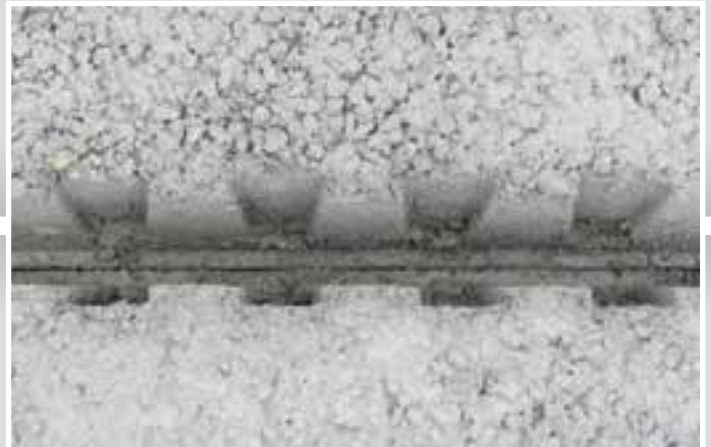
Top view of the joint between the panels. This provides the shear key between the panels, providing a monolithic slab.
